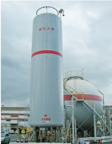
液化水素貯槽 設計圧力: 0.97MPaG 貯液量: 42.3m³ Liquid hydrogen storage facility Design Pressure: 0.97MPaG Liquid Storage Capacity: 42.3m³
